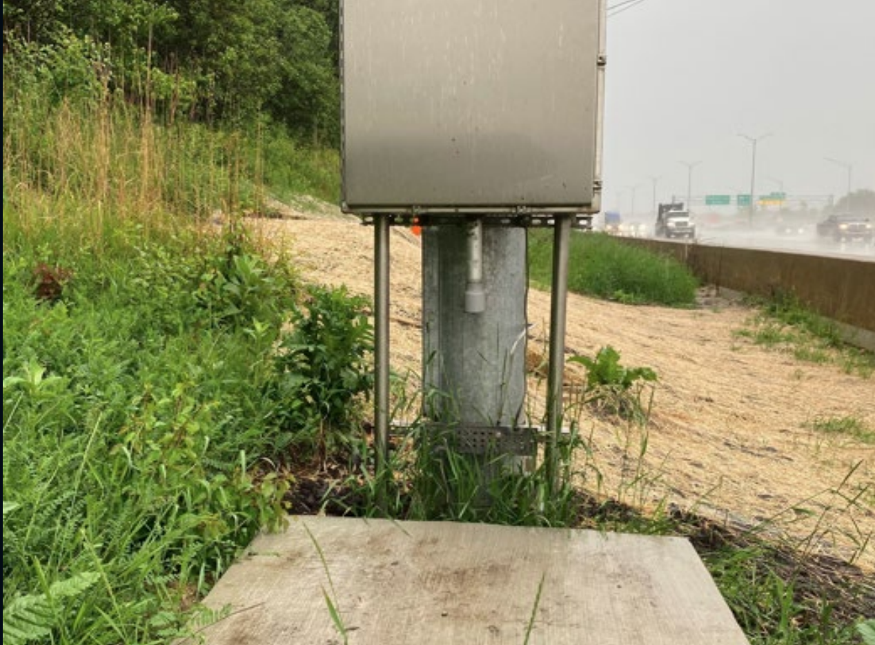
ITS Enclosure with Type A Concrete Foundation
