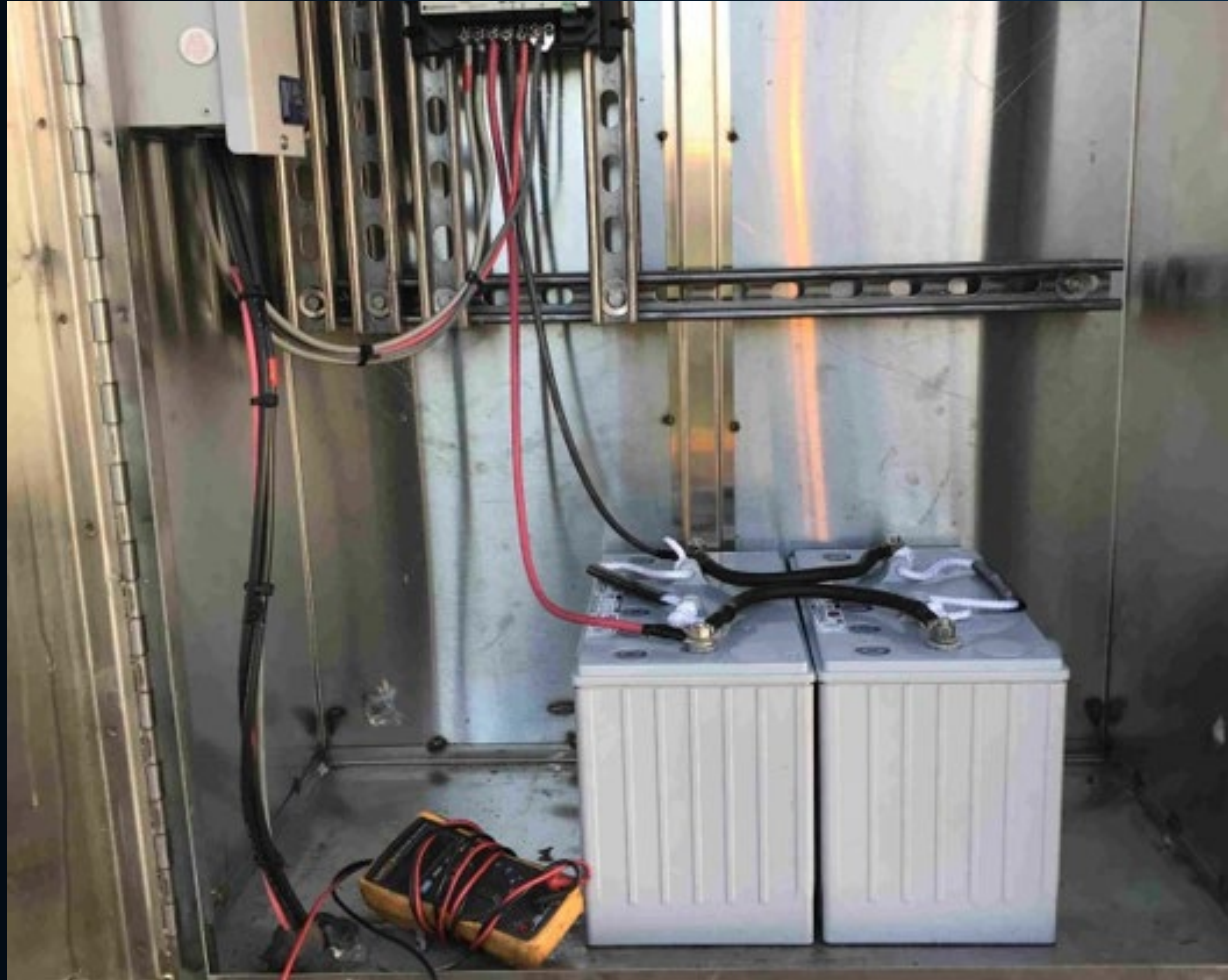
Old Batteries to Dispose per Regulation
