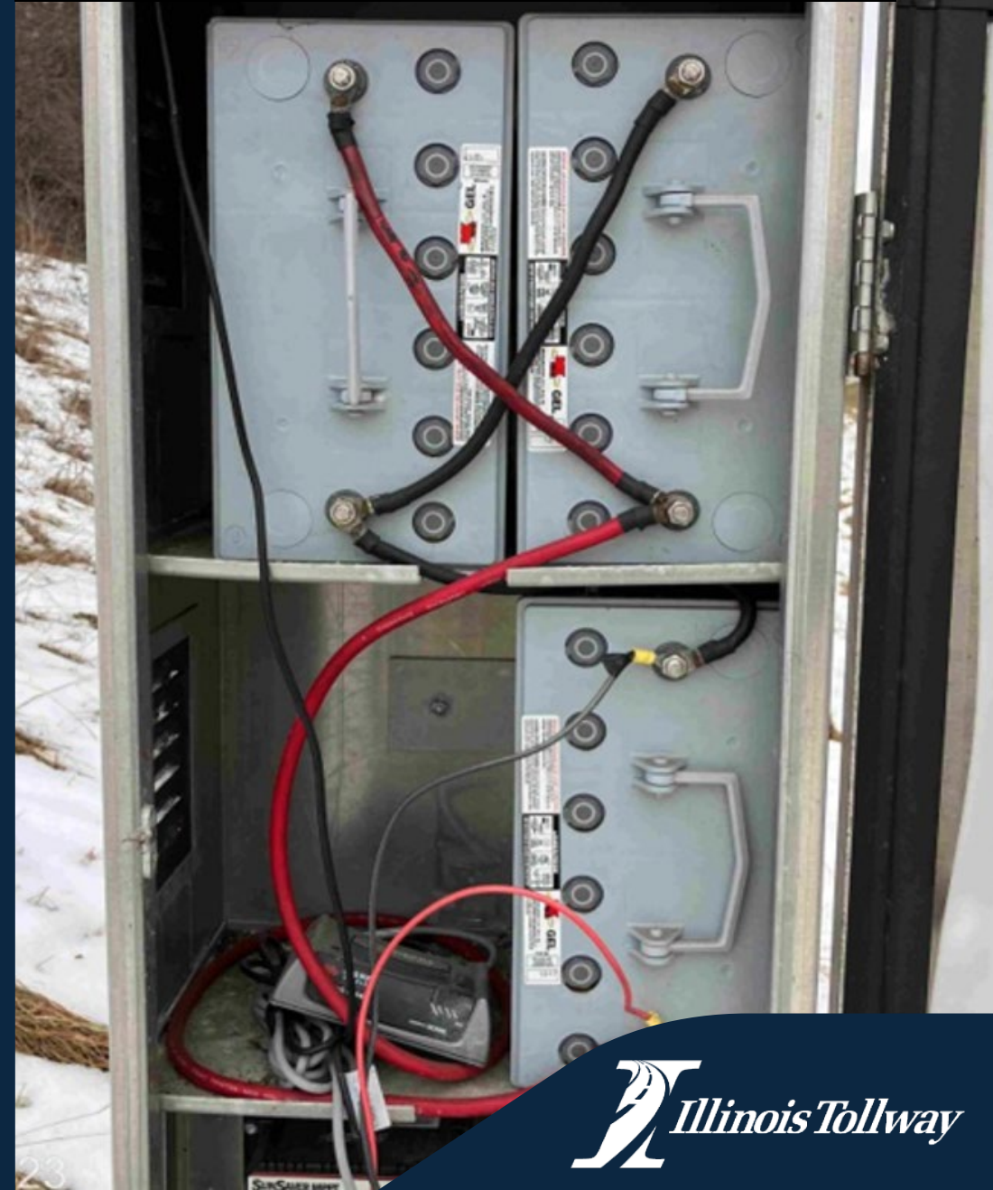
Battery Box/Modem and Power Converter Enclosures
