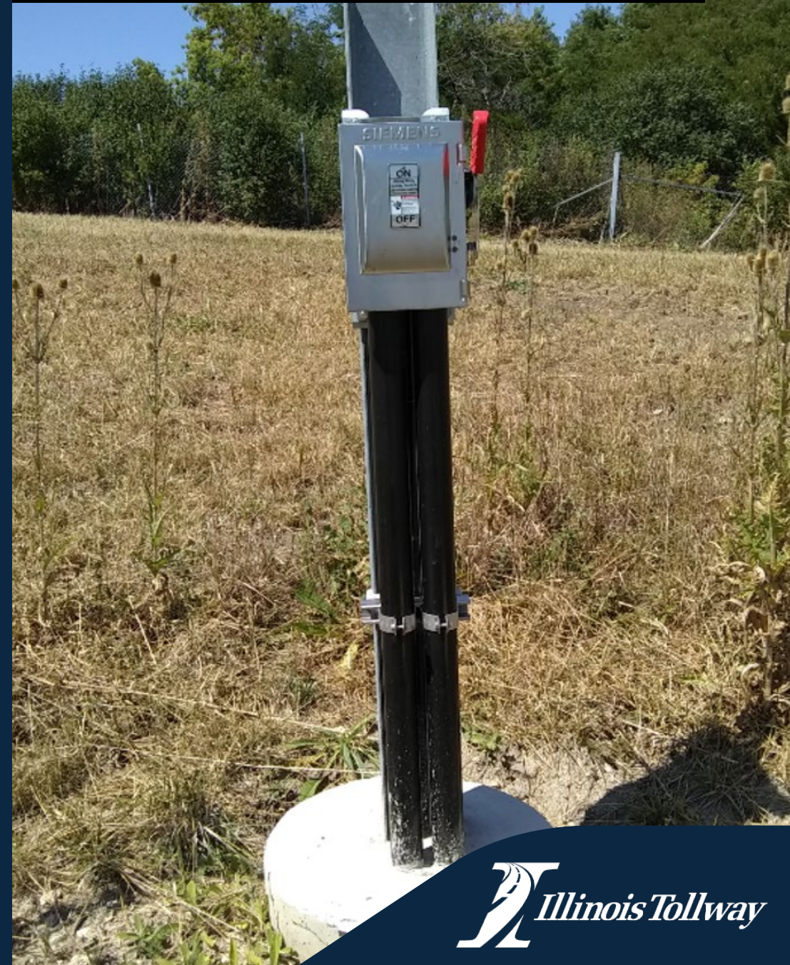
ITS Disconnect Switch installed upstream of ITS Pole
