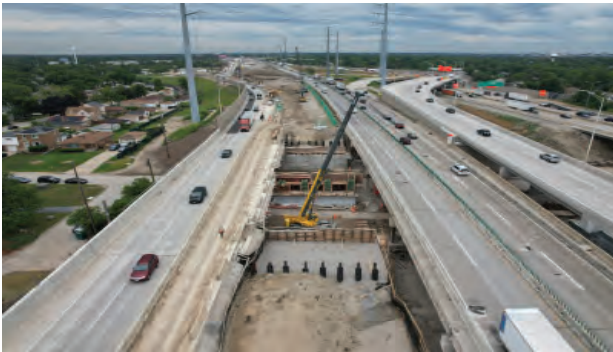
I-290/I-88 Interchange Project at I-294 progress at I-290 facing south near Berkeley.
